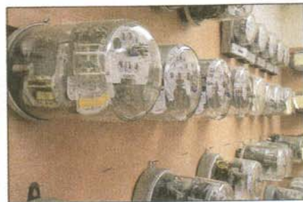
Meters in the new metering test room.
